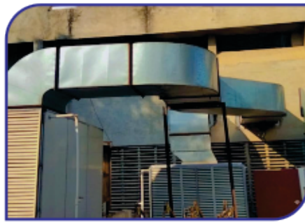
Air Cooling GI Ducting
