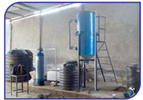
ETP / STP PLANT
