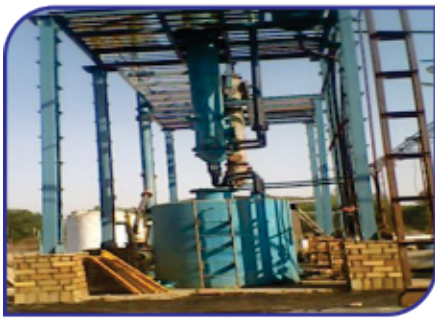
PP FRP Scrubber Column
