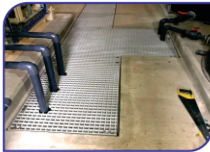
Gutter Line Frp Grating
