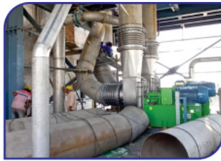
MS, SS, GI Pipe Line
