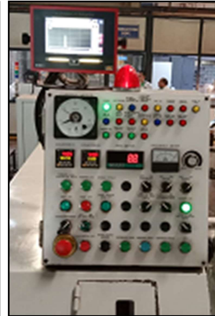
Sensor panel Installed over the machine panel.
